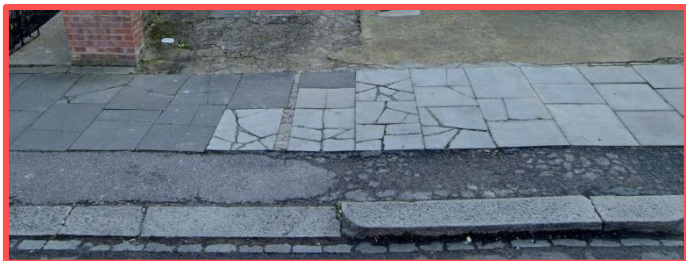
A 'red' condition concrete flag footway in Barnet
