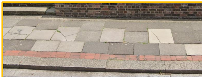
An 'amber' condition concrete flag footway in Barnet
